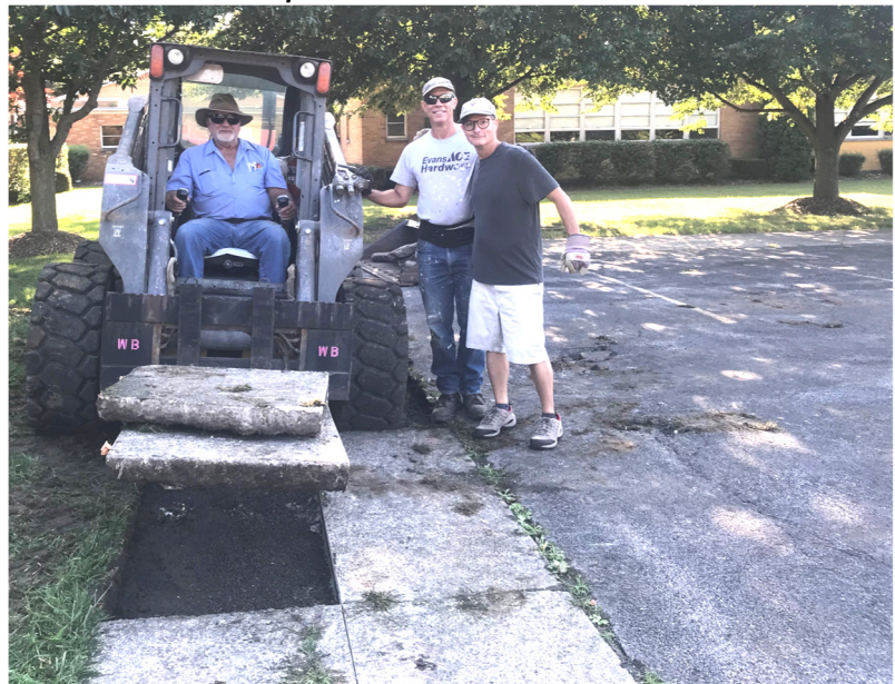
Thank you to Don Kreher, Jim Richardson (not in the picture), Mario Candino and Steven Flumerfeldt for all their hard work removing old concrete so that new can be poured!
